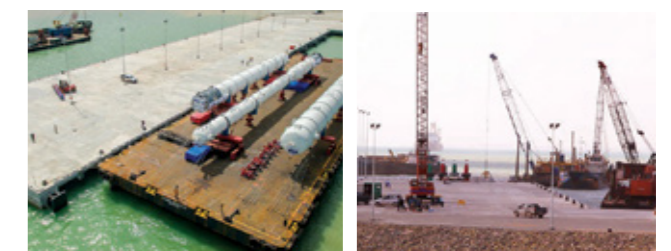
Unloading large process equipment in one of the Material Offloading Facilities in Pengerang, Johor
